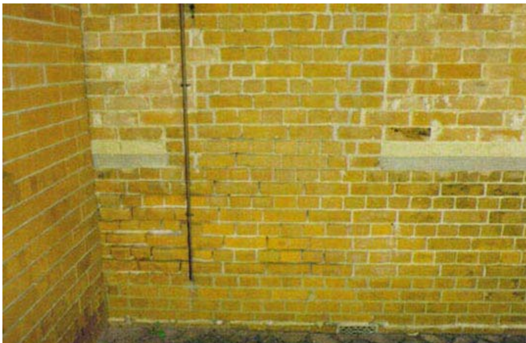
Plate 4: General view of Lectros (LE) panel, exterior face. Note salt attack at lower level and location of downpipe.
