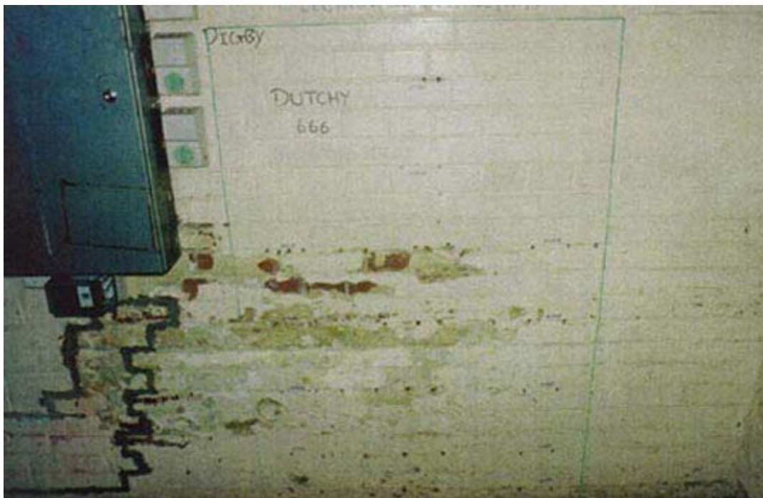
Plate 1: General view of Untreated (NT) panel. Note Lectros control unit below distribution board.
